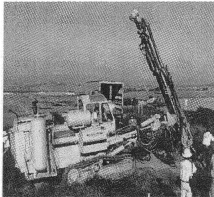
Fig. 5. Drilling for the installation of the monument legs at station BILL, located at the Metropolitan Water District's facilities at Lake Skinner. This station is named for Bill Young, who is a volunteer contributor to the SCIGN project and member of the EC. The principal of these monuments is to anchor deeply into a large volume of ground at a depth of 12' to 30' while decoupling from the surficial 12' of soil that is most likely to creep. It is thought that a major contribution to random long-period (>6 mo.) noise in GPS time series is attributable to monument instability from soil creep.
