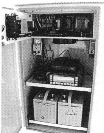
Fig. 6. SCIGN station equipment enclosure.
